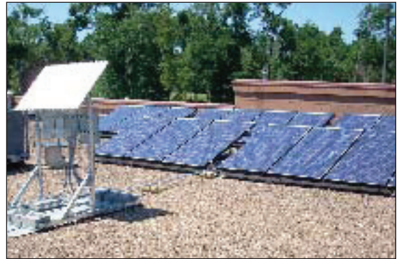
Solar panel system on top of a Jason's Deli location in Beaumont, Texas.
